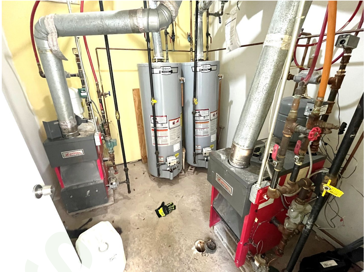
Figure 4 - Boiler room at [REDACTED]
