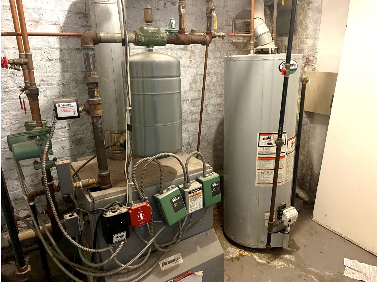
Figure 13 - gas fired boiler and hot water heater at [REDACTED]
