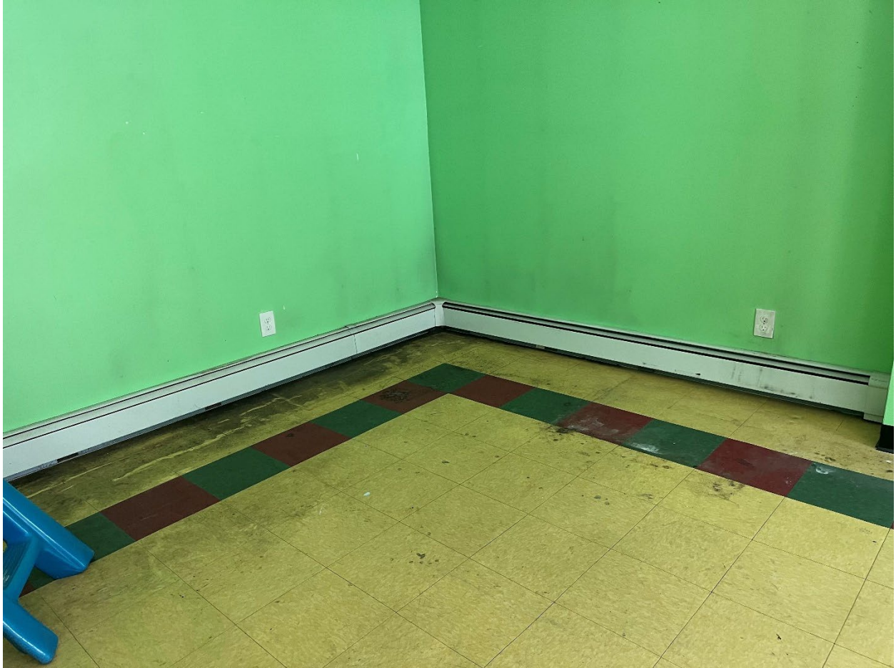
Figure 7 - Baseboard heating at [REDACTED] daycare
