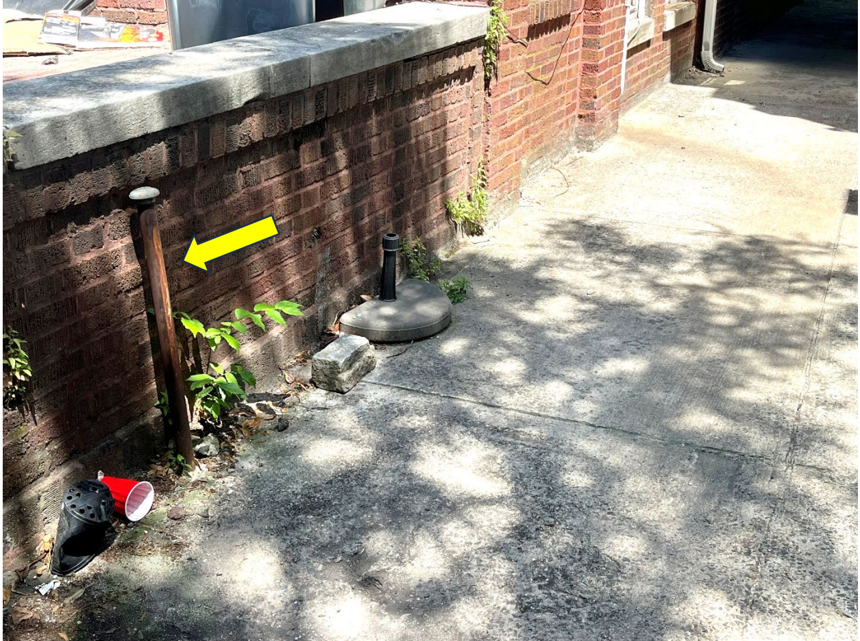
Figure 23 - View of an oil tank vent pipe by [REDACTED] property
