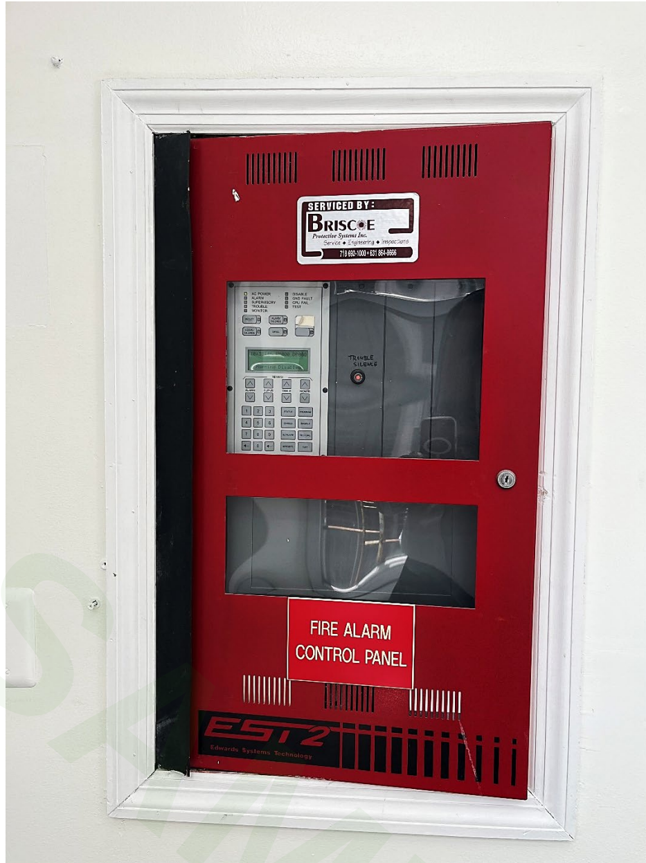
Figure 14 - Central fire alarm system for both buildings
