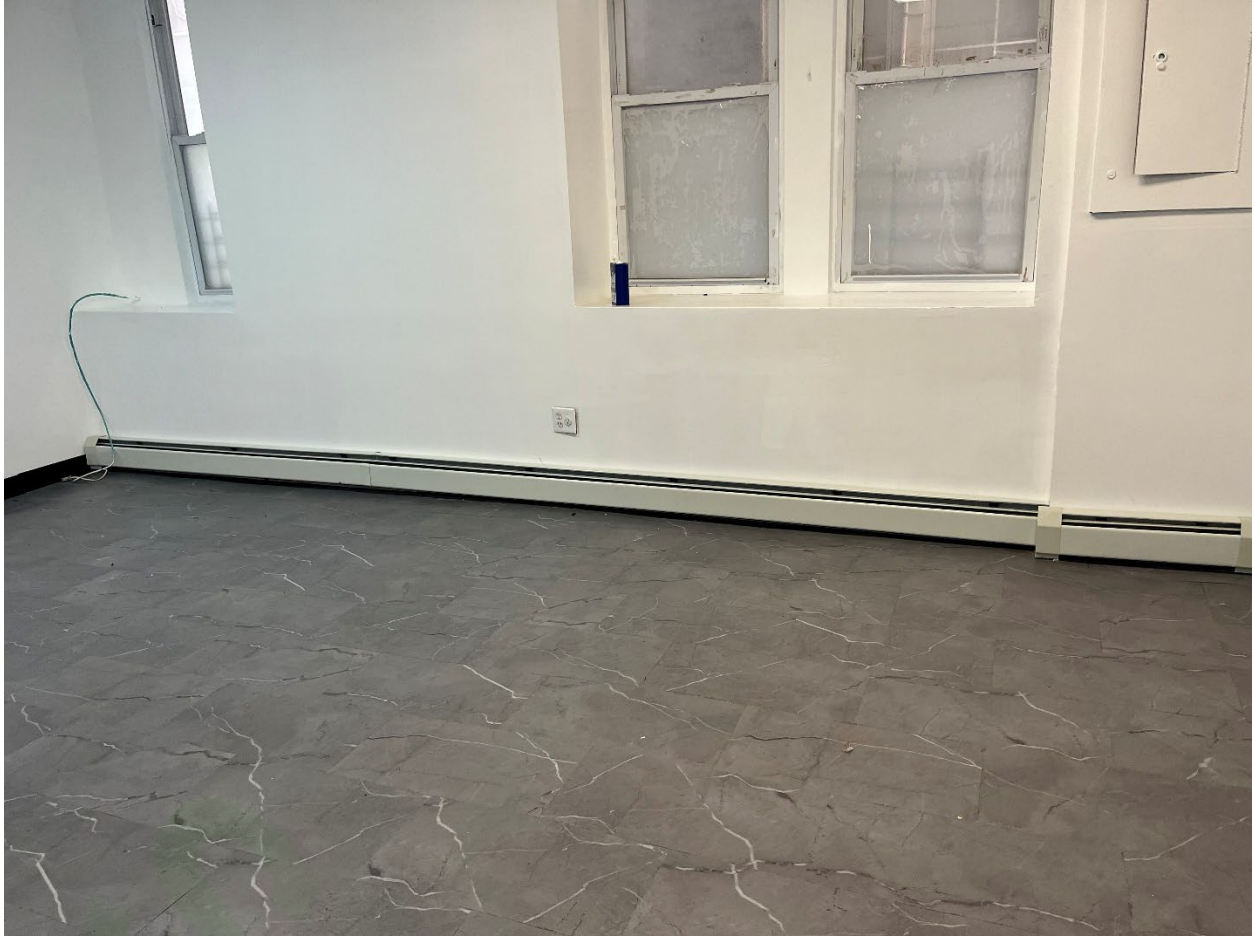
Figure 11 - Baseboard heating at [REDACTED]
