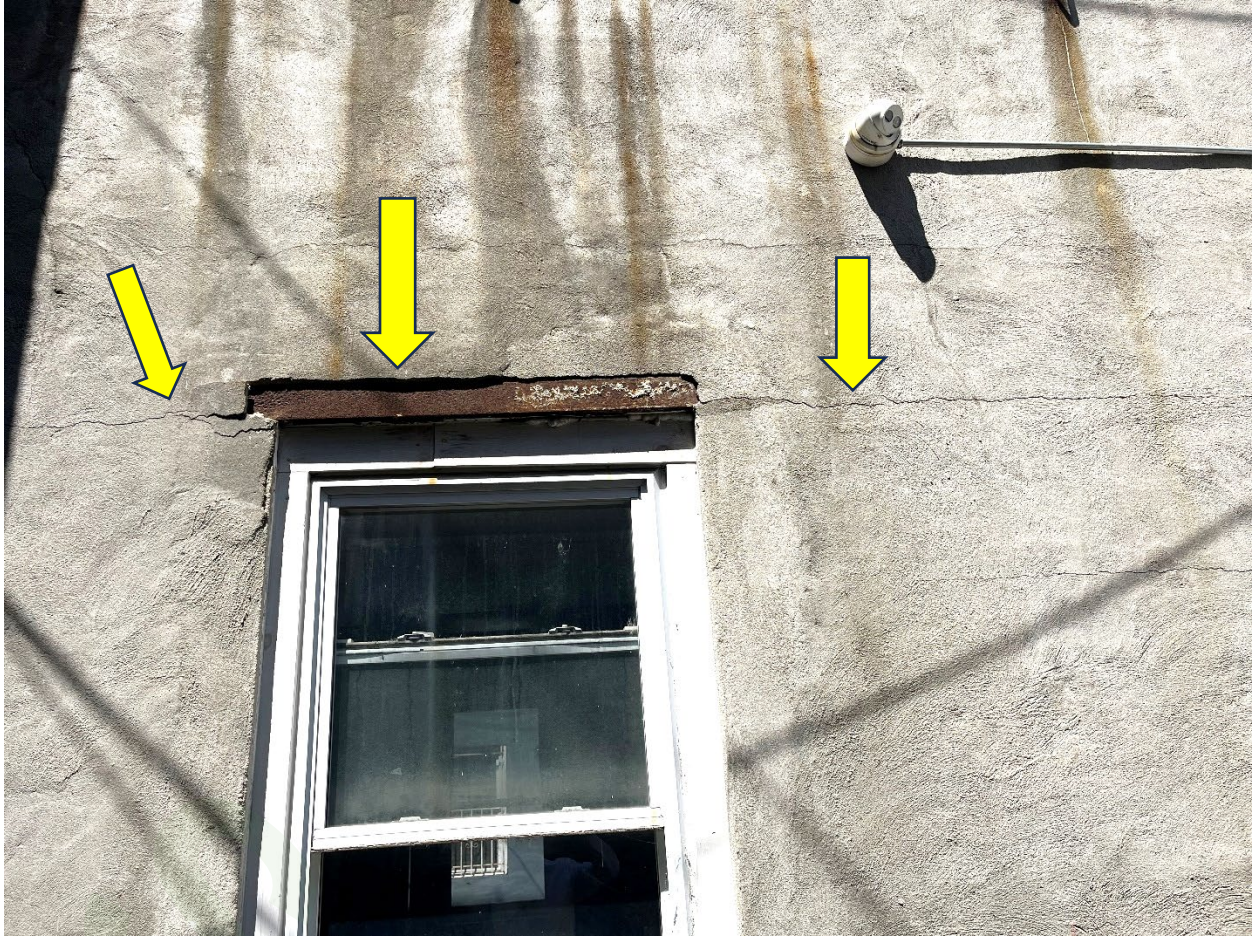
Figure 15 - exterior wall and window at [REDACTED] – requires some repair
